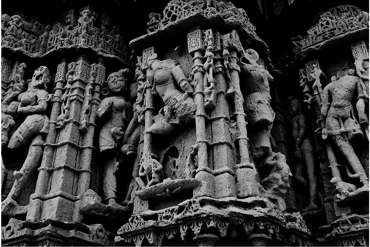
Rukmini Devi Temple, Dwarka, ASI monument number N-GJ-128, showing significant natural deterioration of soft sandstone, as atmospheric erosion has significantly aged the unrestored 12th century structure. Photo Madhuranthakan Jagadeesan, 1 October 2013, Creative Commons Attribution-Share Alike 4.0 International license.
